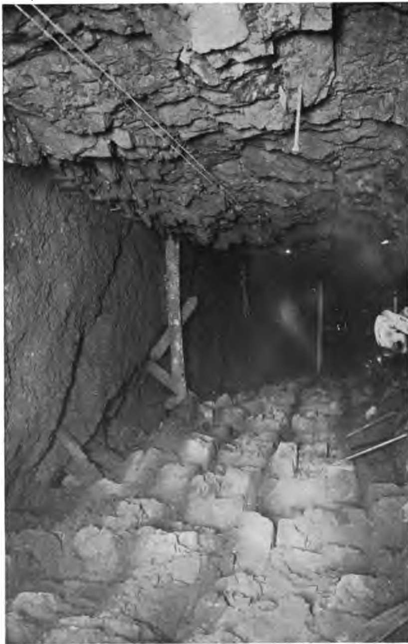
PLATE 90.—Rondout Tunnel in Limestone in which was Found Evidence of Former Caves, now Filled with Clay. Note water-worn roof of clay seams and vertical cracks in limestone.
